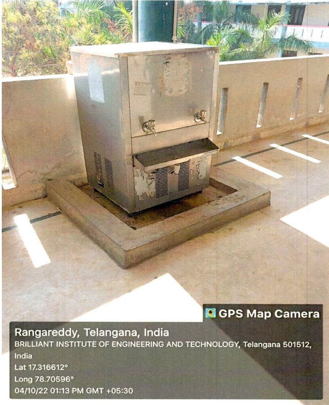
Drinking water facility
