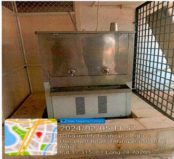
Mineral Water plant
